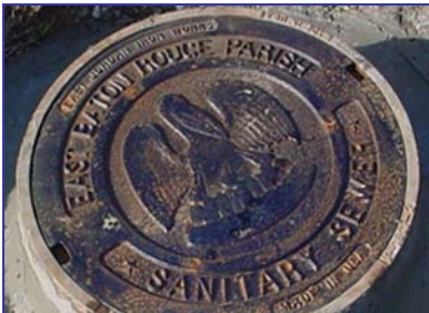
One of the first steps in rehabilitation includes a physical inspection of manholes and pipes to identify blockages.
